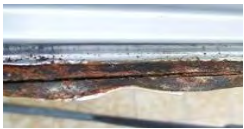
Example of flange corrosion
